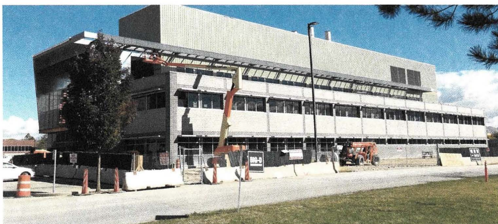
The UDAF Division of Laboratory Services will occupy a portion of the new Unified State Lab in Taylorsville. The new laboratory building will also house the Department of Public Safety Crime Lab, and the Department of Health Medical Examiner facilities.
